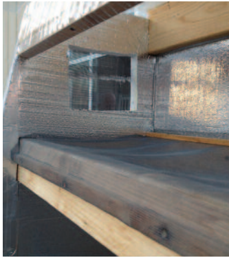
Inside view: insulation and screen shelves
