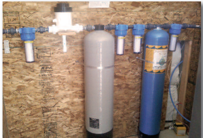
1. Initial installation of Lake Water System.
