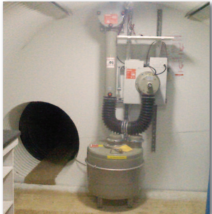
Shelter air filtration system with exit tunnel on left side.
