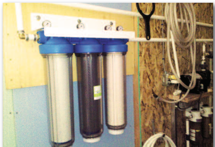
3. Gang filter installed in parallel line flows through UV sterilizer.
