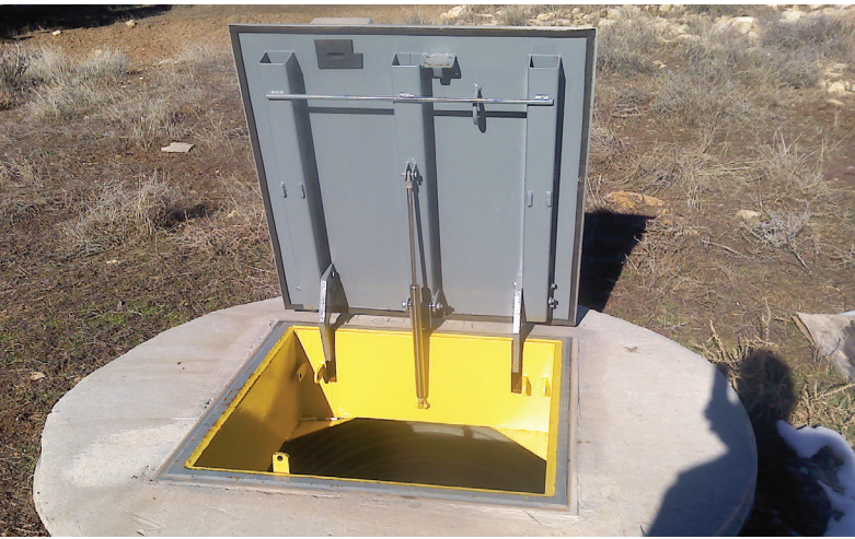
Typical shelter access hatch. Provides security and shelter integrity.
