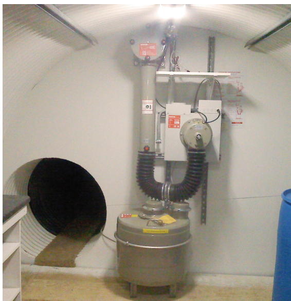
Shelter air filtration system with exit tunnel on left side.
